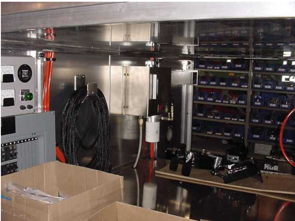
Photo 11 Remote oil reservoir tank w/filter mounted
